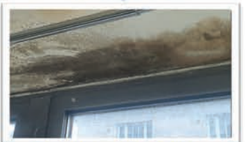
Water Ingress & Mould
