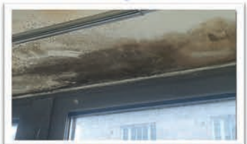
Water Ingress & Mould
