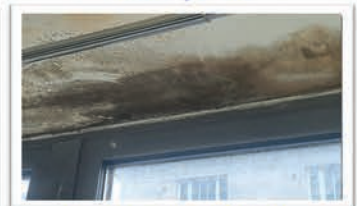
Water Ingress & Mould
