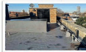
Flat & Commercial Roof Leaks
