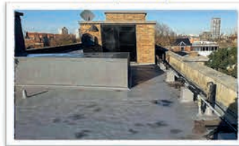
Flat & Commercial Roof Leaks
