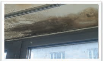
Water Ingress & Mould
