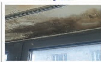
Water Ingress & Mould
