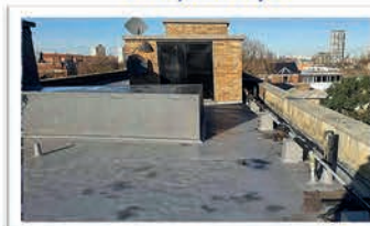
Flat & Commercial Roof Leaks
