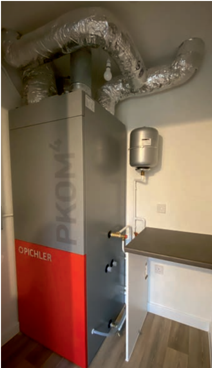
A Passivhaus-certified compact service unit located in a utility room; heat recovery ventilation with two integral heat pumps – one for space heating and one for water
