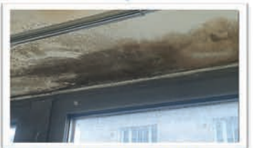
Water Ingress & Mould
