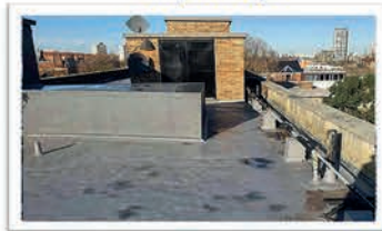
Flat & Commercial Roof Leaks
