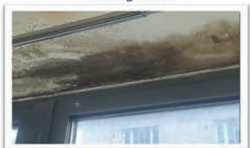
Water Ingress & Mould
