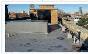
Flat & Commercial Roof Leaks
