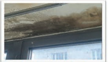
Water Ingress & Mould
