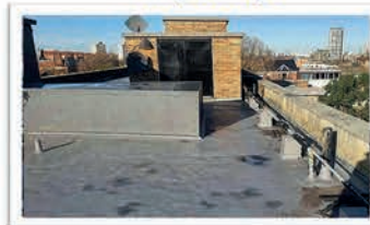
Flat & Commercial Roof Leaks
