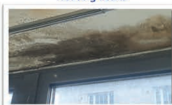
Water Ingress & Mould
