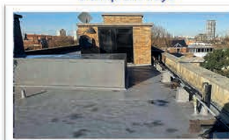
Flat & Commercial Roof Leaks
