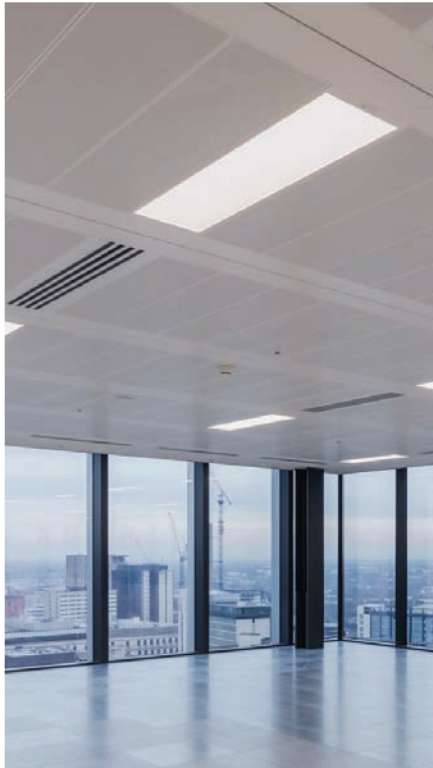
Linear bar diffusers reduce condensation at the BREEAM Excellent 103 Colmore Row, Birmingham
