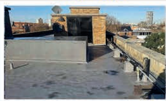
Flat & Commercial Roof Leaks
