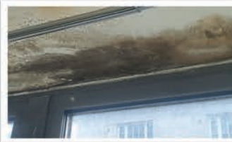
Water Ingress & Mould
