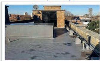
Flat & Commercial Roof Leaks
