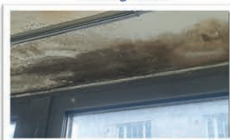
Water Ingress & Mould
