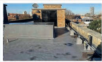
Flat & Commercial Roof Leaks
