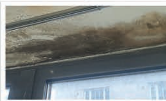
Water Ingress & Mould
